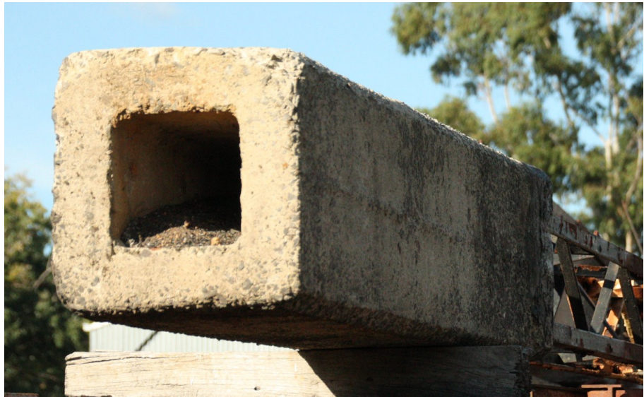
Figure 6 (left). The bottom of a lattice mast foundation showing the lightening hollow. Notice the rough 'as cast' finish of the foundation. Healesville.
