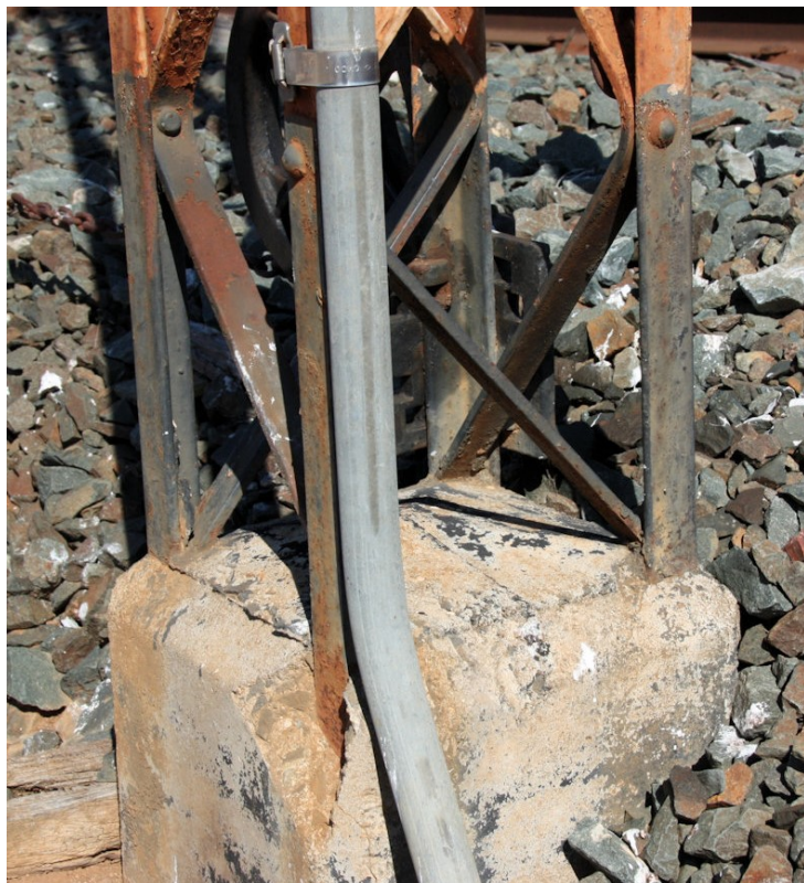
Figure 5 (below). Detail of the foundation the Up Home from the Deniliquin line at Barnes.
