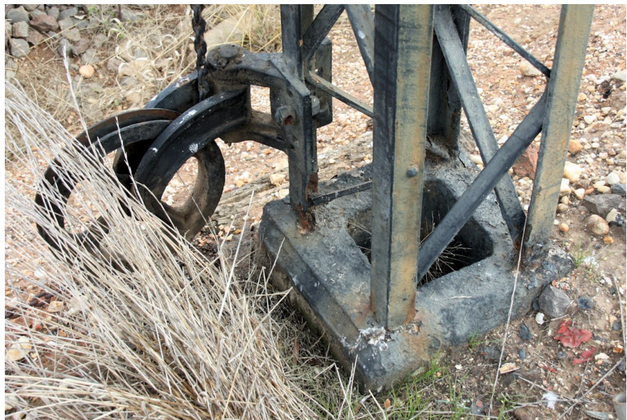
Figure 7. The Up Home signal at St Arnaud had a hollow foundation. Note the sharply defined bevel and the flat top of the foundation outside the line of the angles.
