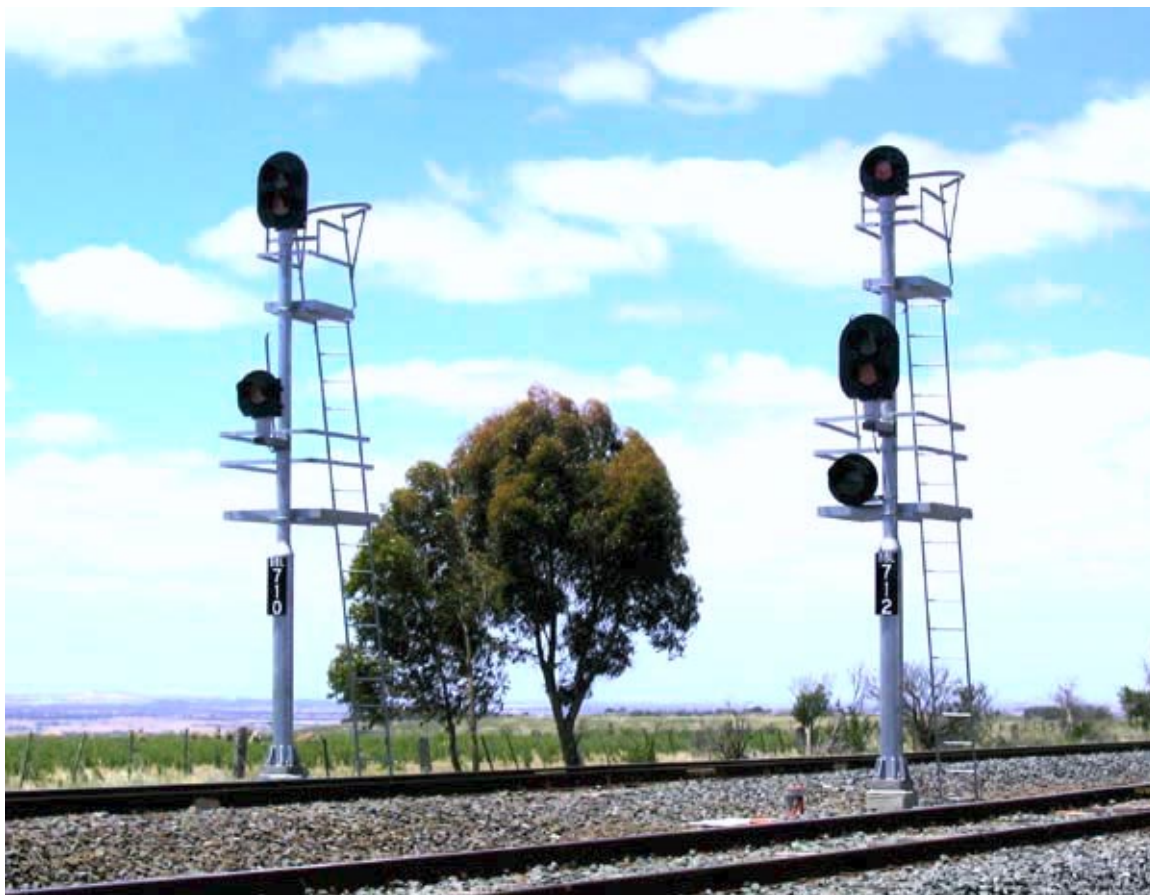
The new Up Departure Home signals from Bank Box loop are typical of the signals provided on the Ballarat line for the RFR works. The masts are welded galvanised steel, and the heads are LEDs. Unlike the new LED signals on the North Eastern line, large and secure access platforms are provided. The third head on post BBL712 is a '65' indicator, not a low speed light.
